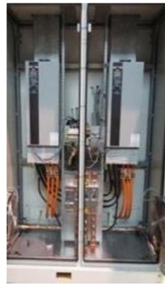
Compressor drives + main power connection
